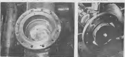
WELDERS ATTACHED this stub to the pipe for mounting the valve and hot tap machine so the cut could be made. WELDERS TA pone un stub na e tubo pa monta un valve y e mashien di hot tap asina cu e cortá por worde trahá.
